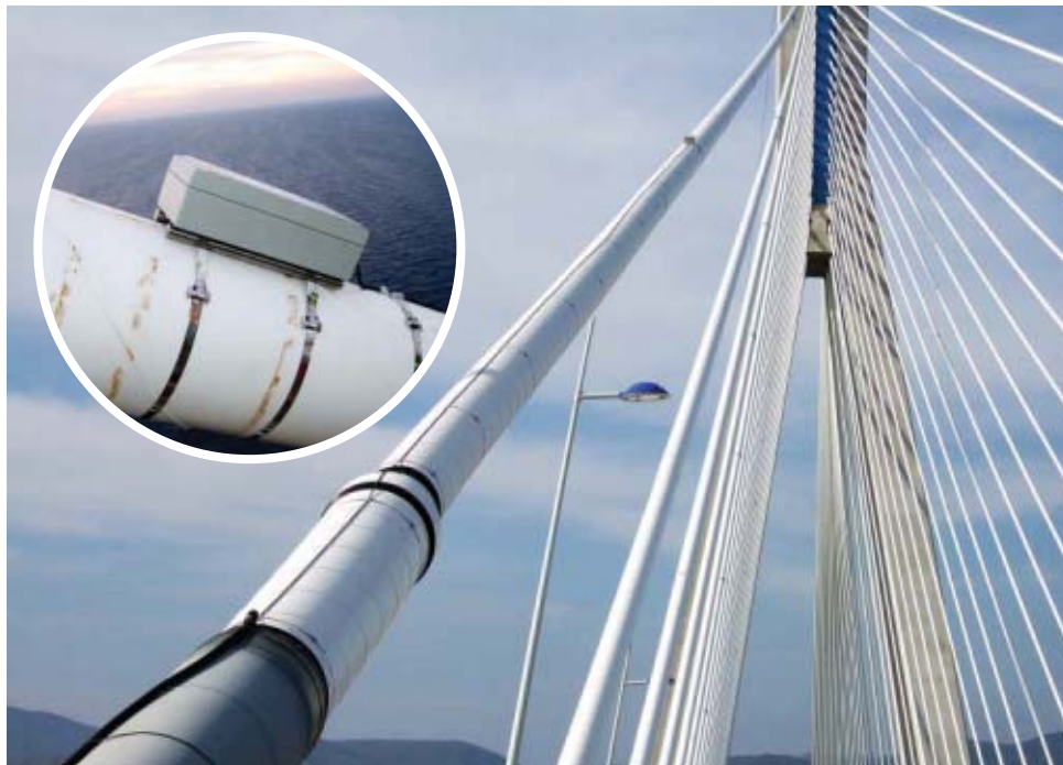
HIGH IQ: Accelerometers, tiltmeters, and strain gauges send their signals to remote engineers. PHOTOS: ADVITAM
